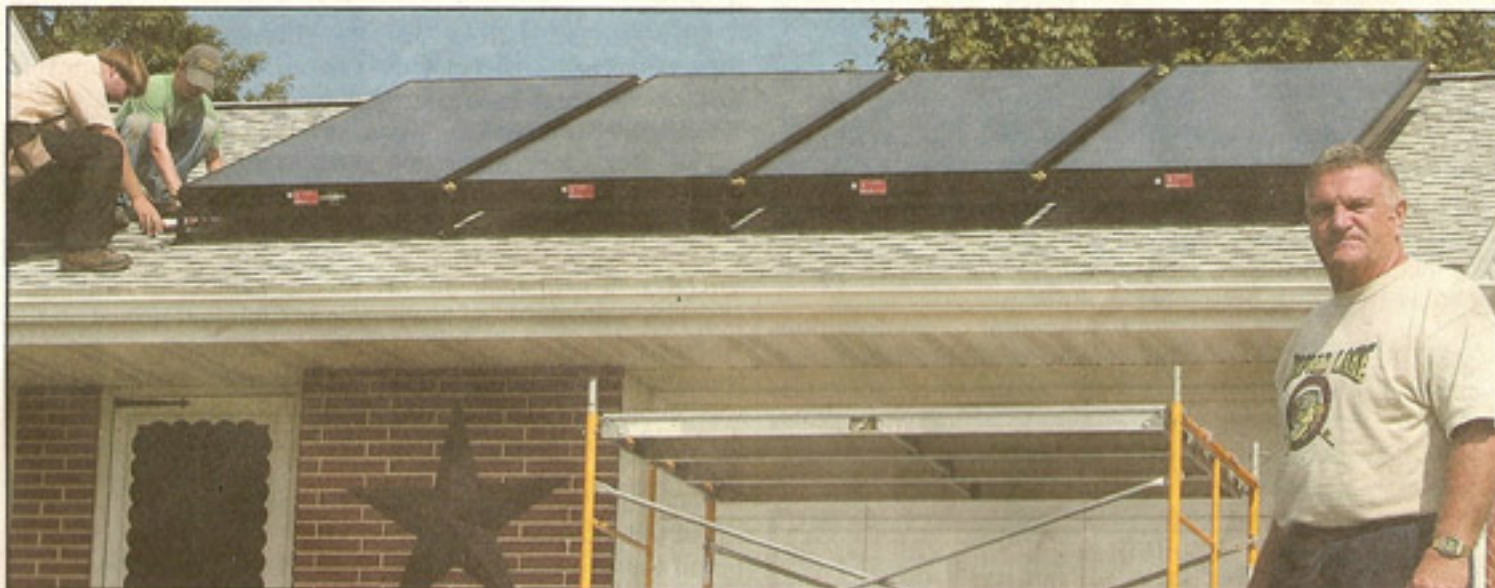
Dan McCardell stands in front of his house on Kirkwood Pike as workers install four solar panels on the garage roof. The panels will help heat the home and provide domestic hot water.
